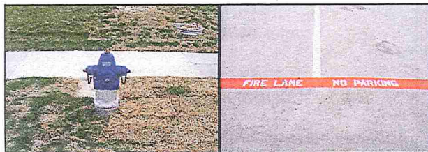
Unobstructed Fire Hydrant
